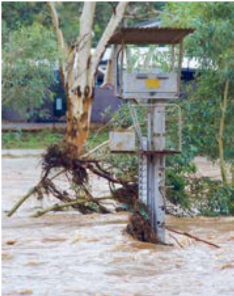
HEIGHT: Flood measuring equipment in the Todd River. (534725)
