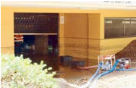
FLOODED: Water being pumped from the Imparja underground car park where several vehicles were inundated. (534725)
