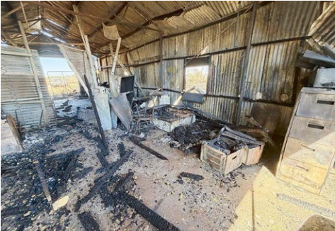
A shed and its contents were destroyed.
