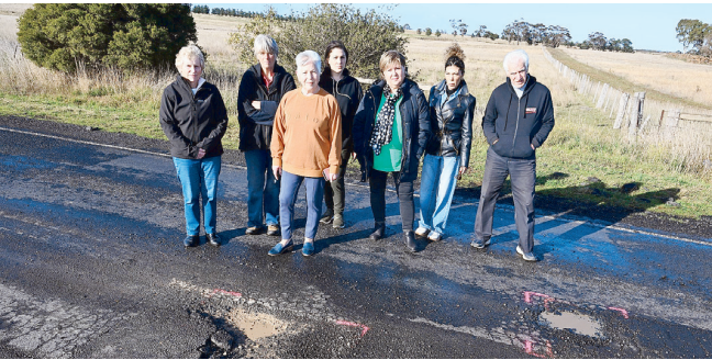
Residents living along Holden Road Diggers Rest are calling on Melton council for a permanent fix of potholes along the stretch of road. (Damjan Janevski) 566651_04
