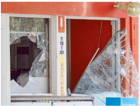
LOOTED: Broken windows at the Shell service station that was looted by rioters. (550927)
