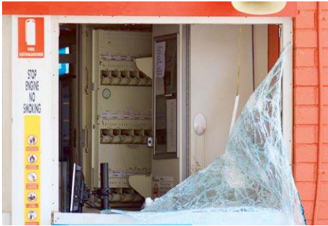
SMASHED: A broken window at the console operator area of the service station that was looted. (550927)
