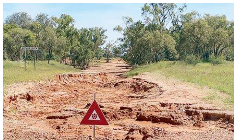
IMPASSABLE: The damaged road surface at the approach to the Arthur River on the Plenty Highway. (Road Report NT)
