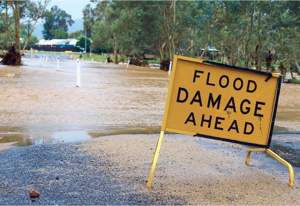
CLOSED: The Tuncks road causeway closed due to flooding and road damage. (Phil Williams: 537763)
